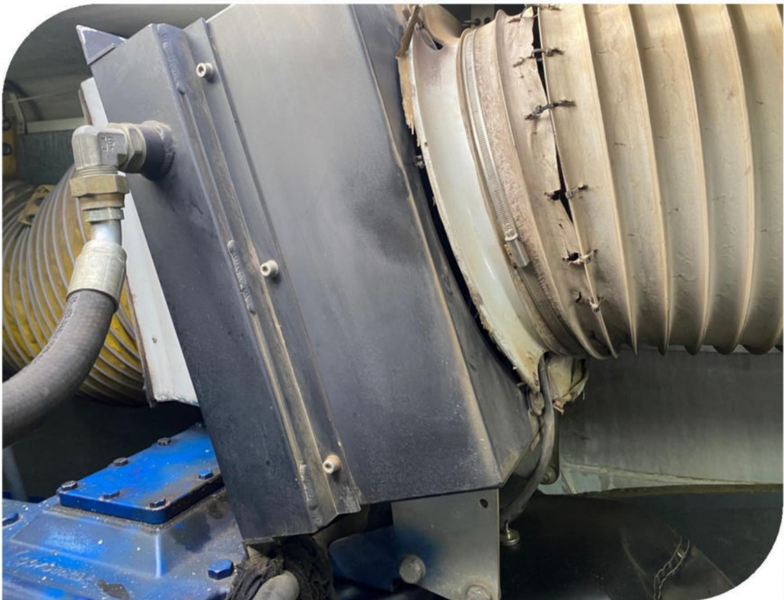
The oil cooling system inside the nacelle
