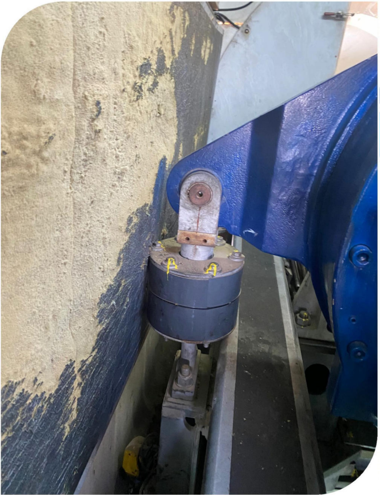
Gearbox torque bracing with damper
