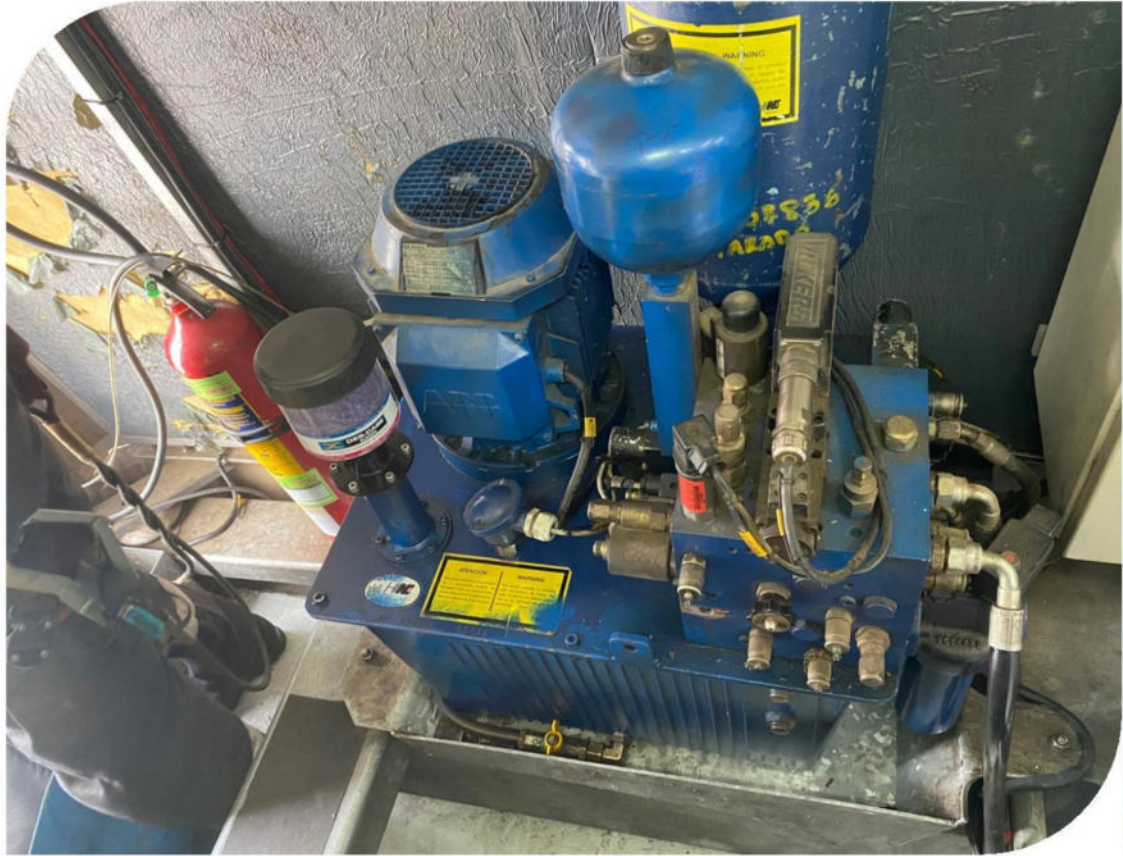
Hydraulic power system
