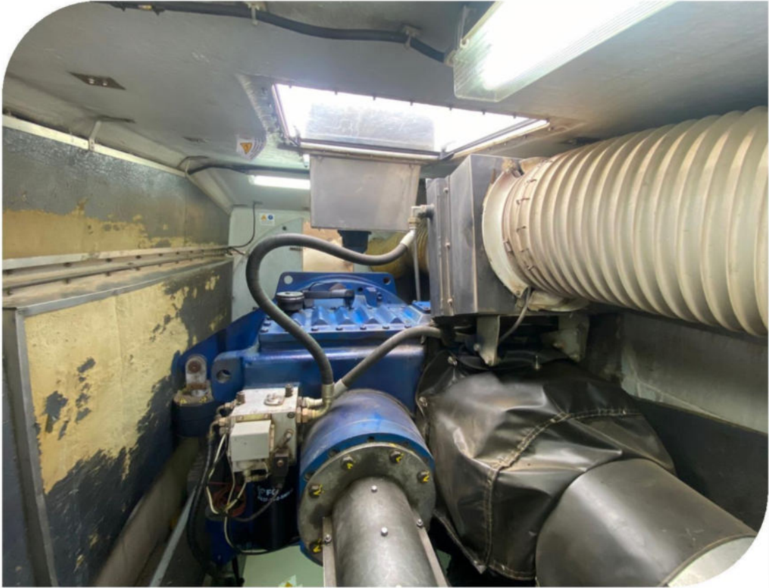
Inside the nacelle, view to the front with Gearbox
