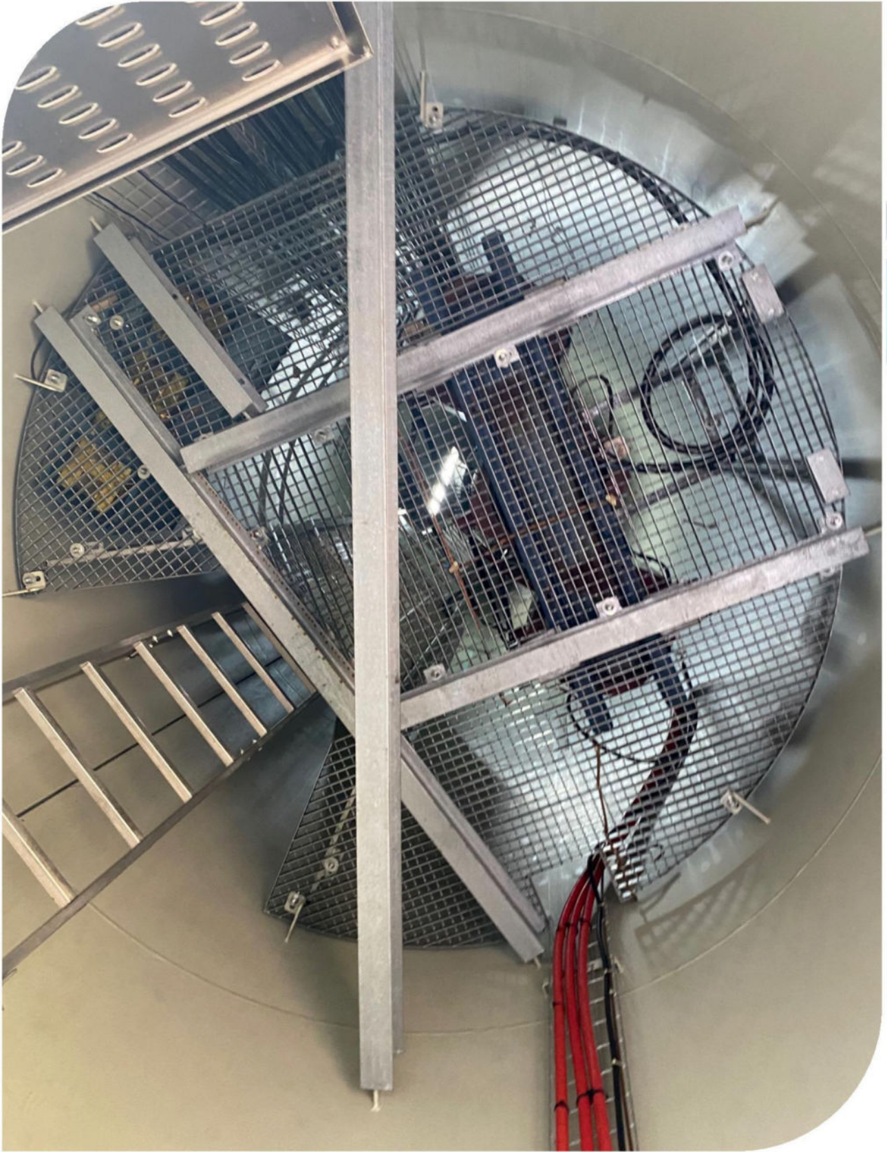
Trafo view from bottom
