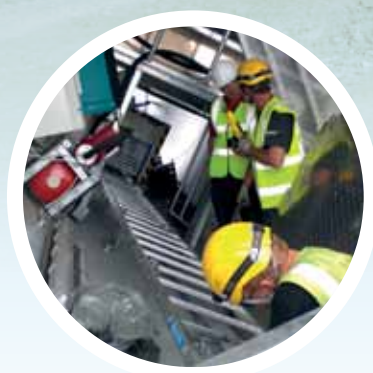
A Latchways cable system is installed.
