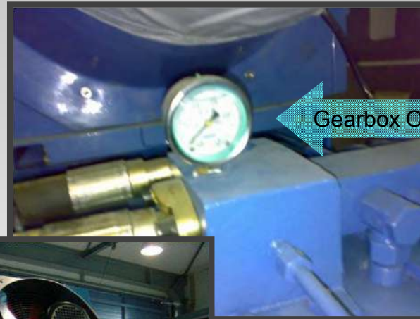
Gearbox Oil Cooling Fan
