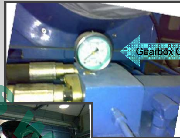
Gearbox Oil Cooling Fan
